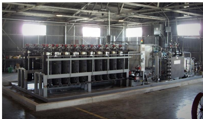
Unattended Oil Polishing Operation of the HERING RCPS® back-end system
