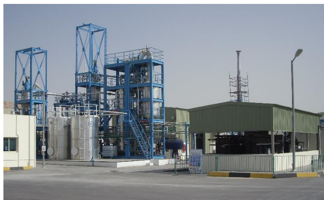
Complete WORP® Waste Oil Re-refining Plant including Front-end and Back-end Systems
